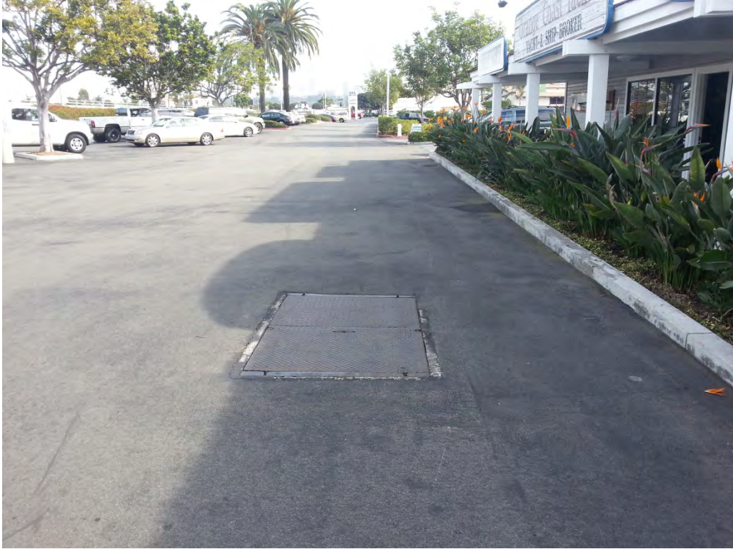
Photo 5: View of utility vaults in front of subject property building, looking east.
